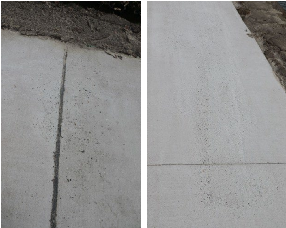
Figure 23 March 2020: Northern and southern side: scaling already visible
