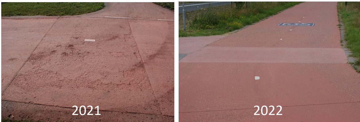
Figure 20 Slabs with most severe scaling have been reconstructed
