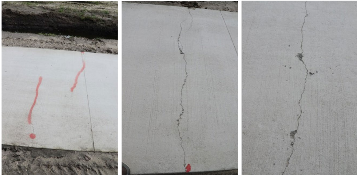
Figure 21 Wild cracks southside, March 2020
