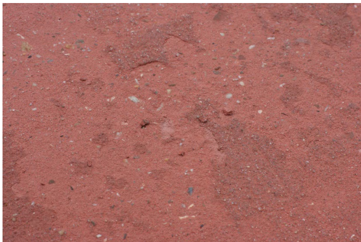
Figure 17 Severe and progressive scaling
